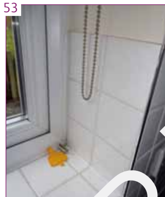
KITCHEN - A wall mounted safety cleat is required to be fitted to secure the window blind cord.
