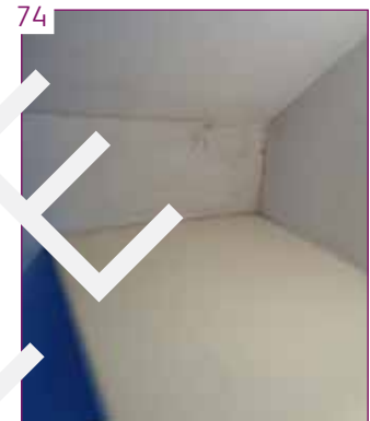
BEDROOM 2 - The left wall to the cupboard is showing signs of damp that needs to be investigated.
