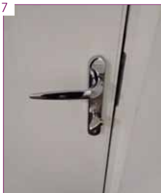
ENTRANCE - Both front door handles working loose.
